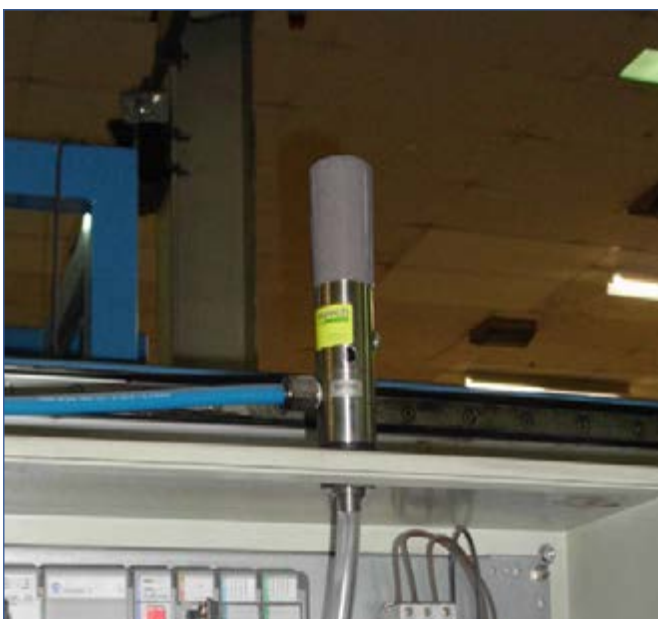
Cabinet cooler fitted to an electrical panel.
